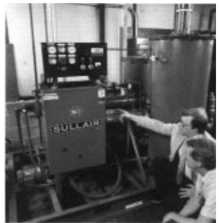
This Sullair Series 20 rotary screw vacuum system is expected to save Hopple Plastics $26,500 a year in vacuum systems power costs. Discussing the installation with Plant Engineer Carl Vollmar is Rick Lee, a representative of the equipment distributor, HRC Compressor Engineering.
