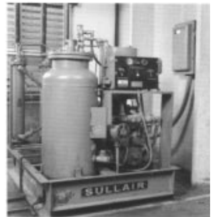
This 12-year-old, 100 hp Series 25 air compressor at Hopple Plastics has run far more than 75,000 hours and continues to operate with its original air end.
